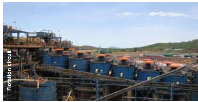
Mill Plant and power generators
