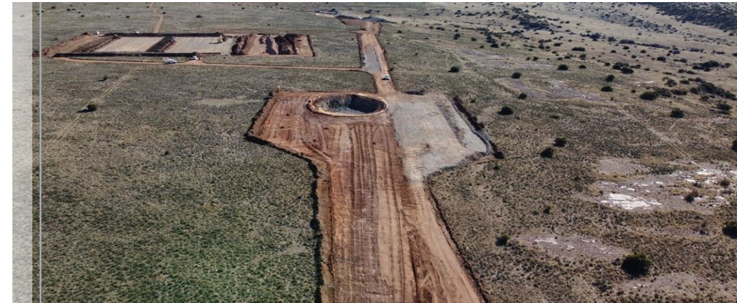
Aerial views of the construction at the Castle wind energy project during August 2023
