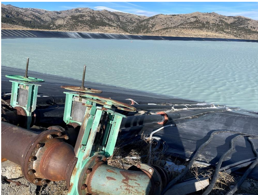
PHOTO 16 – Water reclaim manifold and pipework (November 2023).
