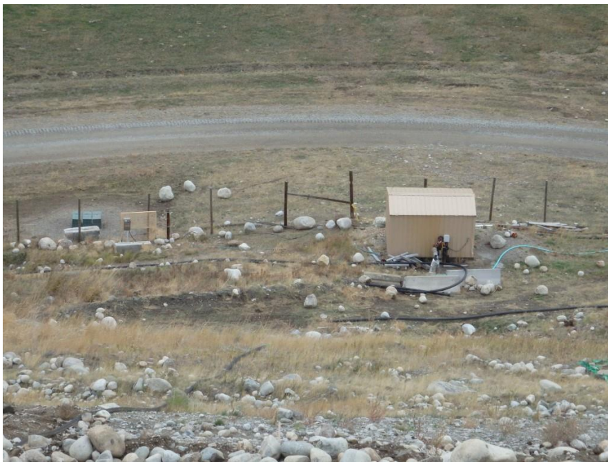
PHOTO 10 – Cell 1 Basin Underdrain Collection Sump and pumphouse (2015).
