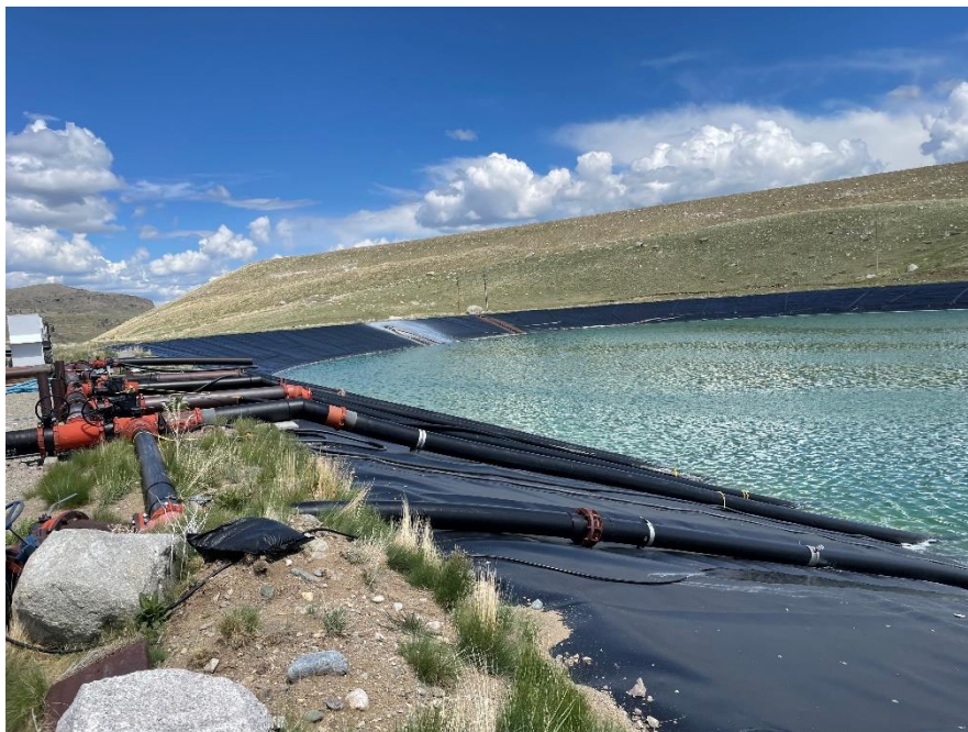
PHOTO 20 – LAD Storage Pond reclaim pipework and pumps (2022).
