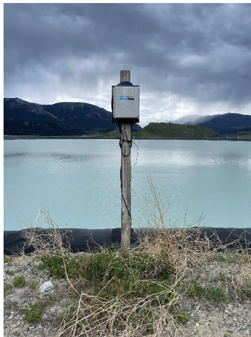
PHOTO 8 – Stage 3 vibrating wire piezometer readout location (May 2024).
