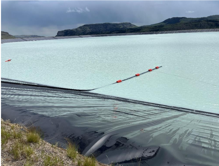
PHOTO 9 – Floating tailings discharge spigot (May 2024).
