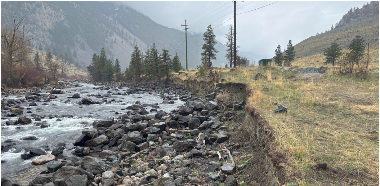
PHOTO 10 – Stillwater riverbank adjacent to East Embankment downstream toe, erosion extents from June 2022 flood event (April 2025).
