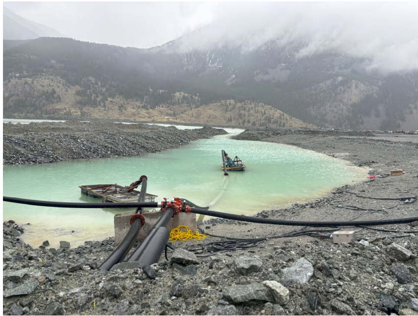
PHOTO 3 – Initial Runoff Collection Sump arrangement (April 2025).
